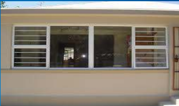
Windows and Burglar Bars
